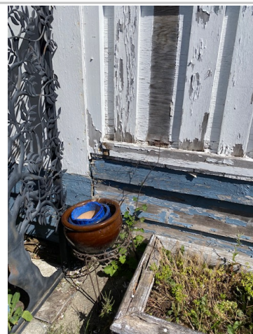
L1-2. Exterior blue and white paint. Lead containing.
