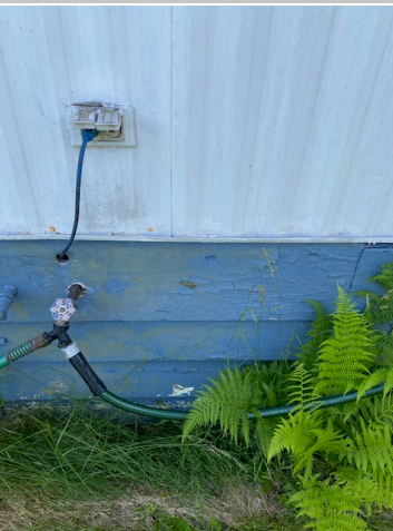
5. Black mastic sealant around exterior power socket. Asbestos was detected.
